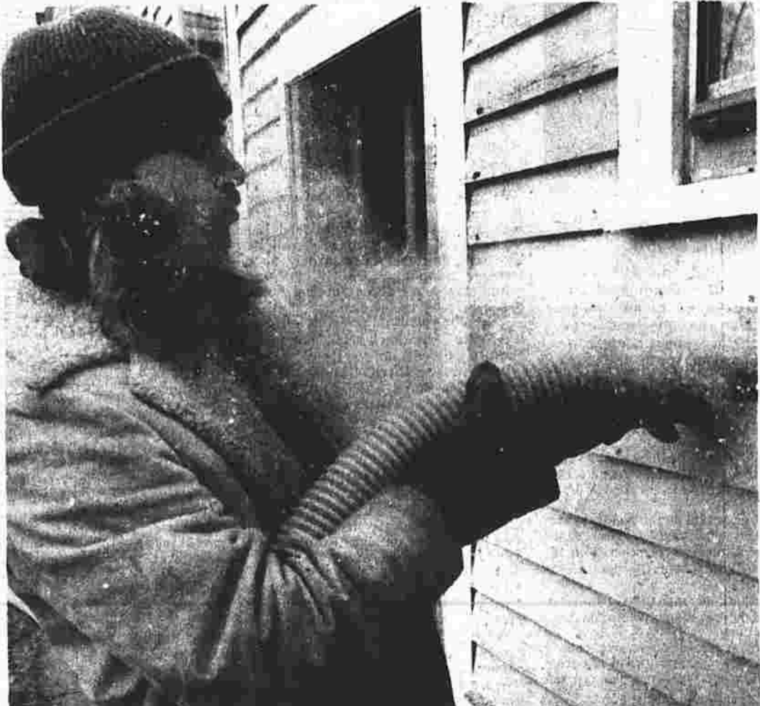
Shelter from the storm The calendar may say it's almost spring, but today's cold and impending snow is enough to remind us it's never too late to insulate the home. Allen Ringstone of Manchester, of the B.A. Lozier Co., races the snowflakes today, as he blows cellulose insulation into a home at 142 Bissell St.
